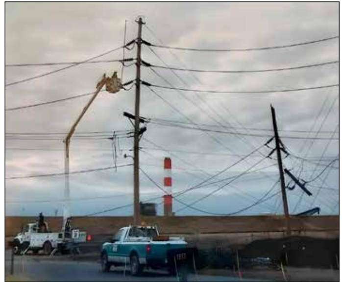
Overhead lines were shredded from the ice storm.
